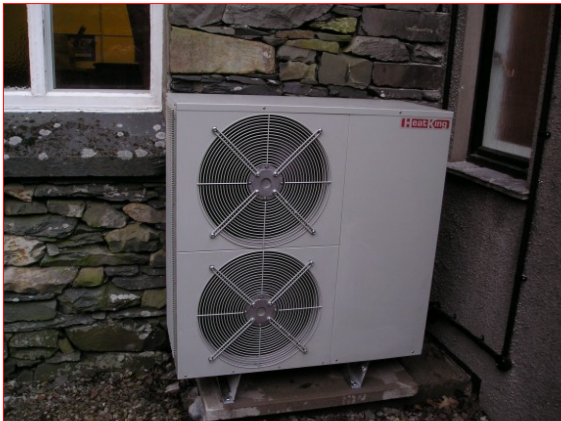
12 kW Air Source Heat Pump at High Wray
