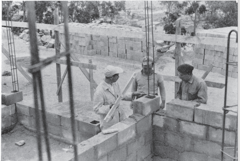
Above : the future owner working on the construction with a professional builder
